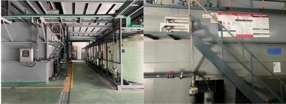
(PGTEX carbon fiber workshop nitrogen, high salt wastewater facilities)
