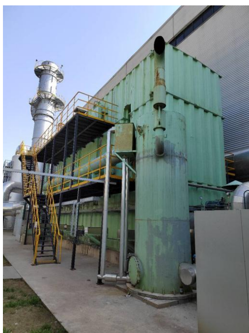
(Grade 5 RTO incinerator equipment)
