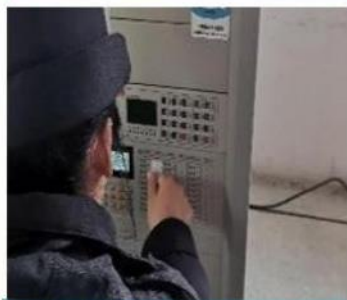
5. After the fire control duty officer confirms the fire situation, start the fire sound and light and fire broadcast
