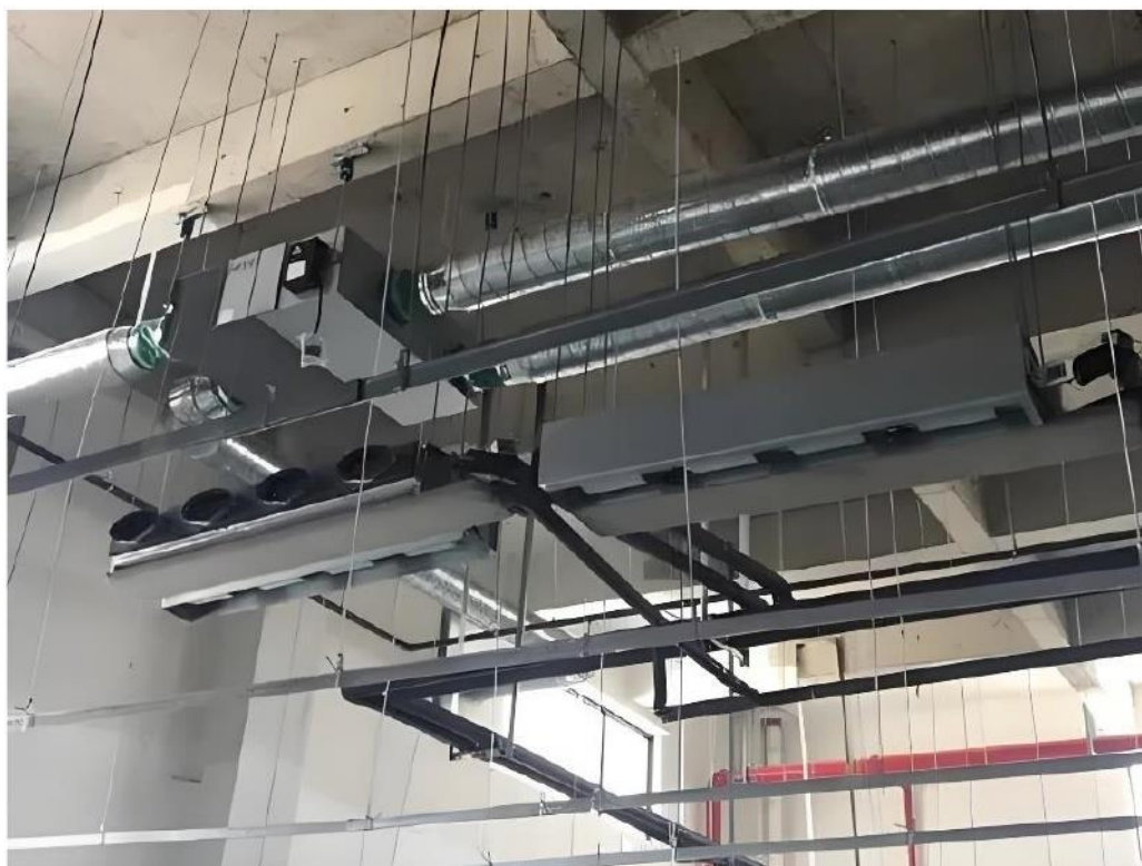
(Air conditioning and fresh air system in workshop)
