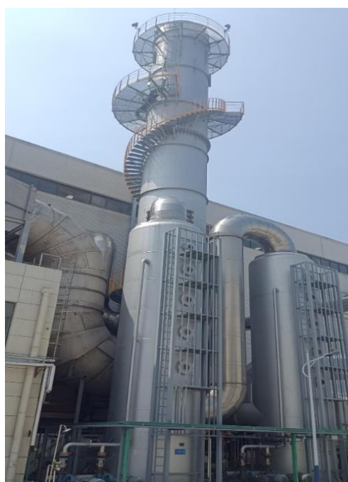
(High altitude discharge of treated exhaust gas)
