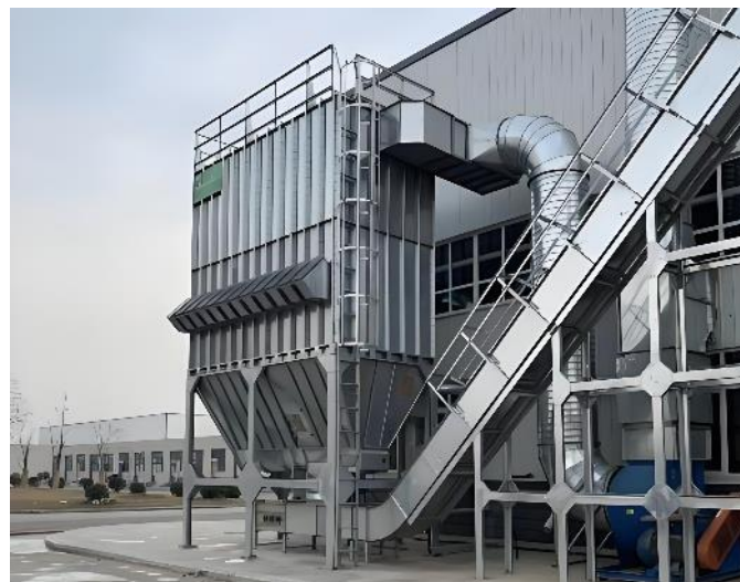
(PGTEX pulse activated carbon filtration system)
